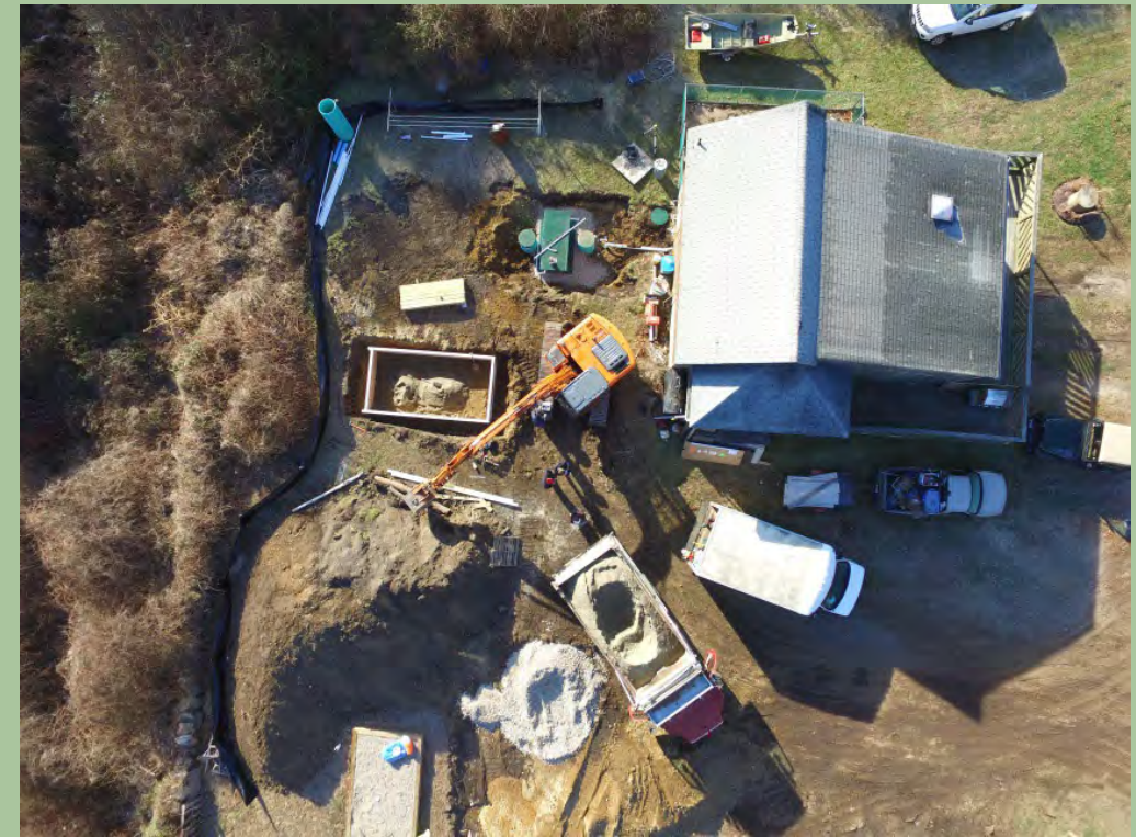
Nitrogen reducing OWTS installed to replace substandard systems located less than 100 feet from a coastal wetlands under the Charlestown EPA SNEP Grant
